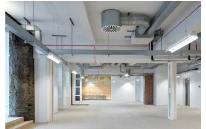
A key driver underpinning the scheme is to expose and enhance the historic fabric of the existing building to create character speculative office floorplates.
